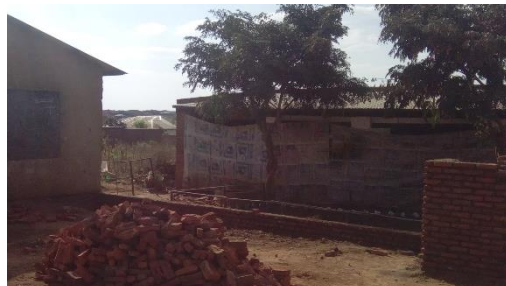
Foundations complete, bricks delivered, bricklayer on the way... New classroom for 100 pupils
